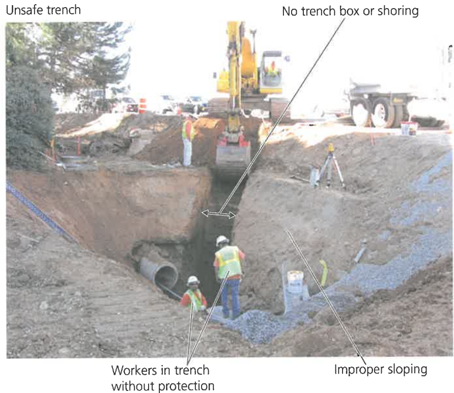
FIGURE 4 Construction site fall hazards
