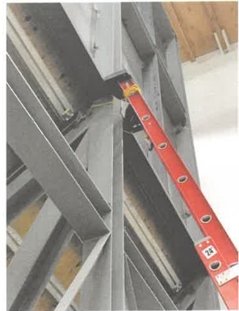
FIGURE 40 Ladder secured at the top
