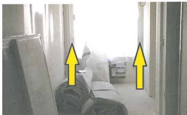
View of window opening from inside building with arrows pointing to brackets that held up guardrail
