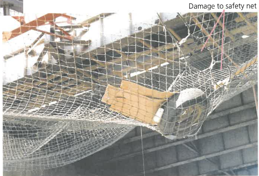
FIGURE 35 Damage to safety net
