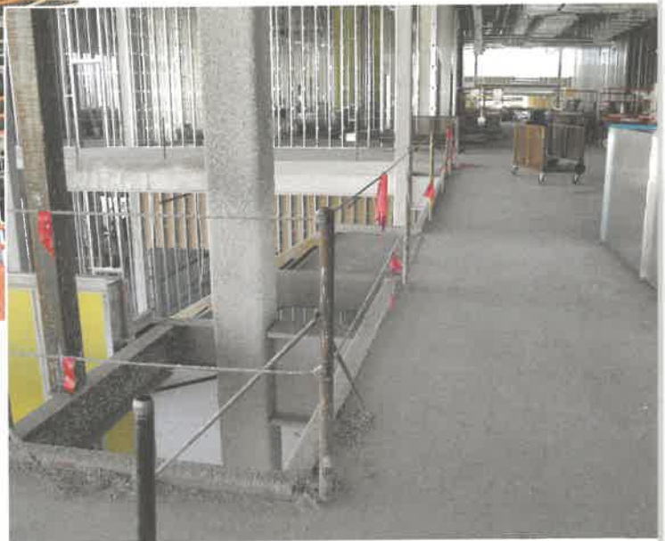
FIGURE 17 Flagged wire rope
