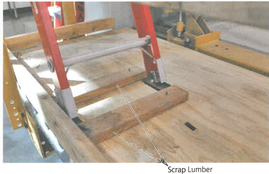
FIGURE 28 Secured ladder base
